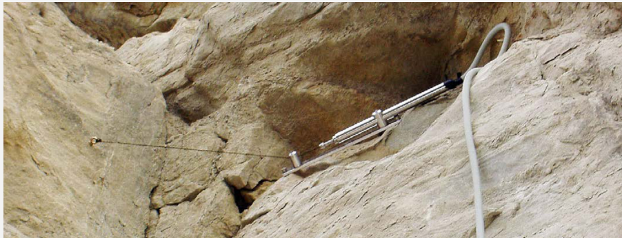
Electrical deformeter installed on a rock fall
